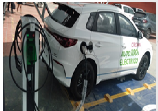
Electrolinera Centro Comercial Mall Ventura
